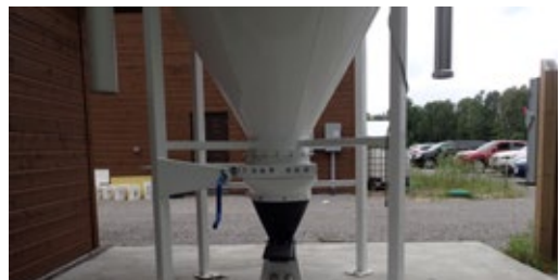
Figure 33. When the boiler's pellet hopper runs low, pellets are automatically delivered from the bulk storage silo shown above via vacuum hoses to refill the hopper.
