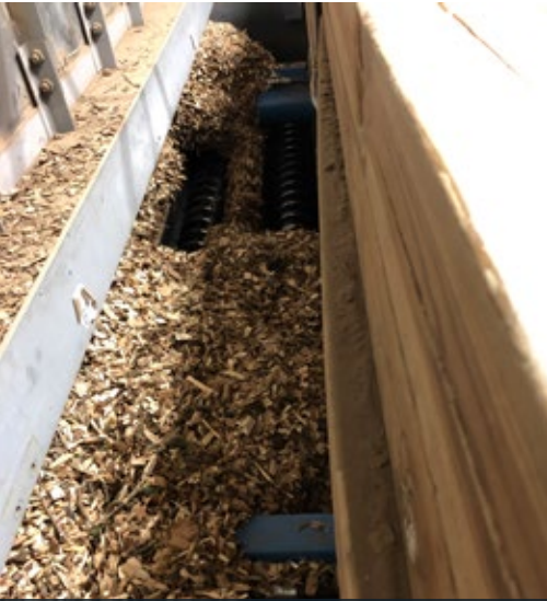
Figure 28. A series of augers automatically feed the chips to the boilers when there is a call for more chips from the boiler's control system. (Photo: Biothermic)
