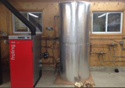
Figure 16. A 30 kW cordwood boiler used to provide heat for a home or small office building. On the right is the hot water storage tank (2 250 L) used to store energy and increase system efficiency. (Photo: Biothermic)
