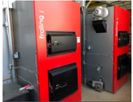
Figure 17. Wood chip boilers installed at Confederation College. Each boiler can provide 500 kW of baseload. These boilers provide 85% of the space heating needs of the 400 000 square foot facility. (Photo: Biothermic)
