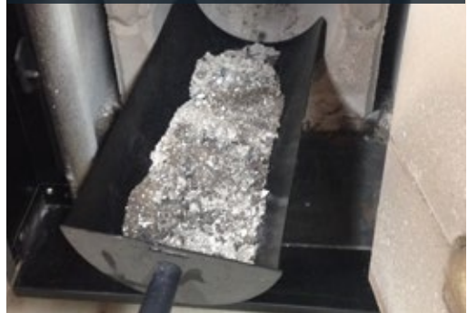
Figure 22. Ash removal systems in combustion systems are user friendly. This cordwood boiler ash removal system uses a custom-designed scoop to easily and cleanly remove ash. This type of system would be typical for the smaller systems used in homes and smaller institutional and commercial spaces. (Photo: Biothermic)
