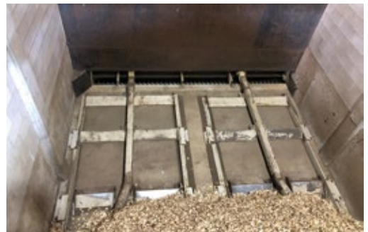
Figure 27. An aerial view of the chip holding room at Confederation College, engineered by Evergreen BioHeat. The scraper floor shown moves the chips along the room's length to a series of augers. (Photo: Biothermic)
