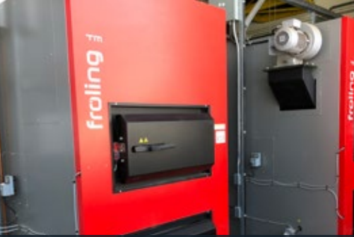
Figure 26. Wood chip boilers installed at Confederation College. Each boiler can provide 500 kW of baseload heat. Together, the boilers provide 85% of the space heating needs of the 400 000 square foot facility. (Photo: Biothermic)
