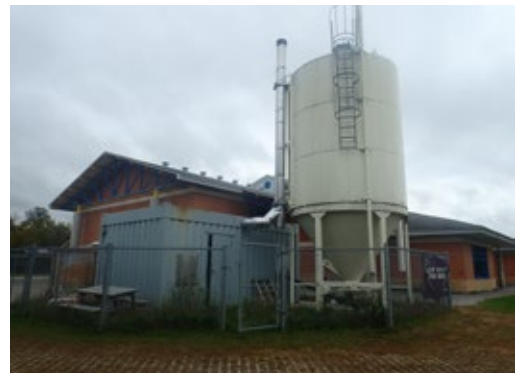
Figure 18. A containerized pellet boiler system with an agricultural silo for pellet storage used to heat a school. This type of containerized system can be used for cordwood, wood chip, and pellet boiler systems.
